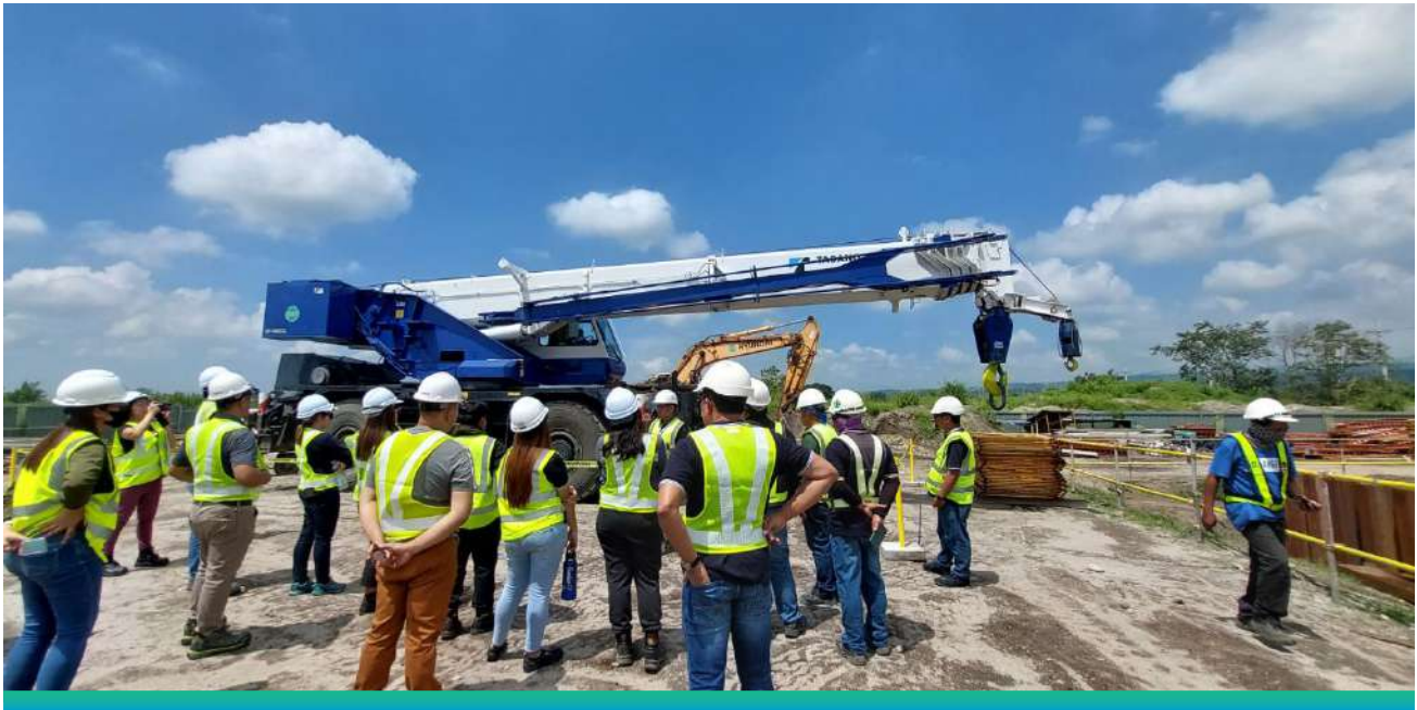
This safety walk-through at our site in Pampanga is just one of the many conducted regularly, aiming to identify potential safety hazards, assess the status of safety in the workplace, and provide feedback to personnel on proper safety practices.
